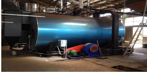
Invercargill Hospital Energy Centre
